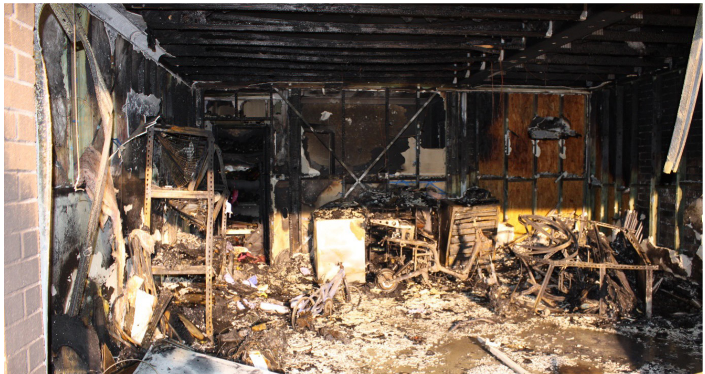
Bike in centre of room is the origin. The cause was failure of the battery pack on charge. Bike was a Fonzarilli electric. House two years new.
