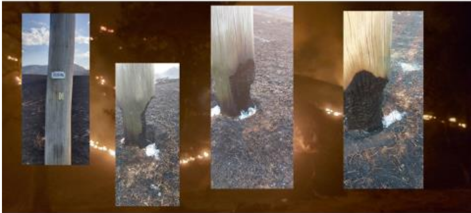
Figure. Electricity distribution system impacted during a bushfire.
